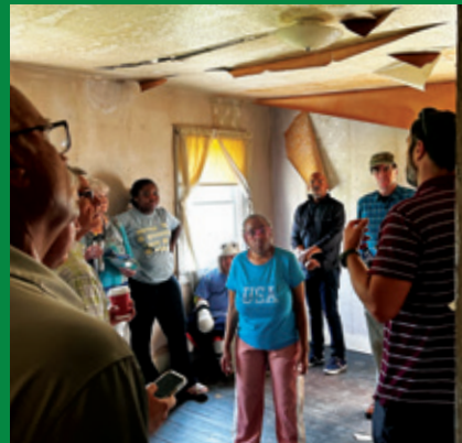
Eileen and others go on a walk-through tour of Reeves Farmhouse before we start renovations.
